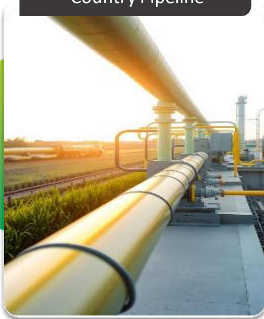
Natural Gas Cross Country Pipeline
